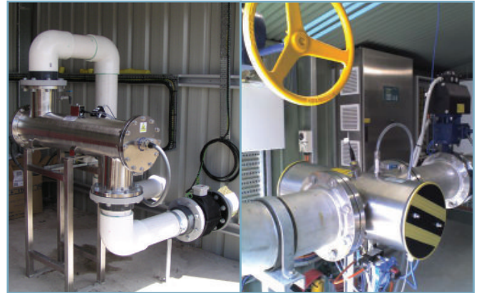
Two smaller “in-pipe” UV systems.
