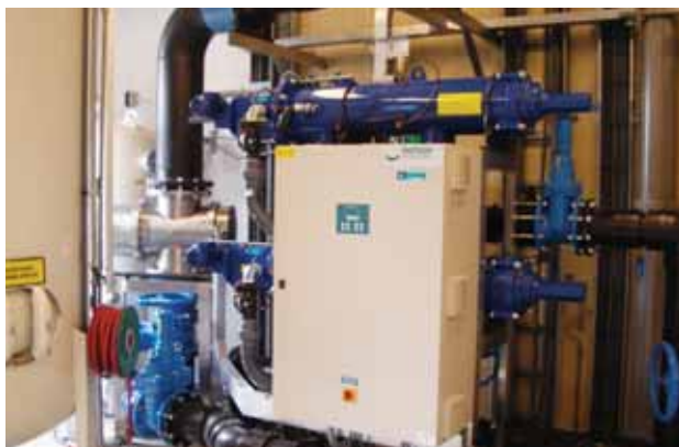
Vlaardingen, The Netherlands, Berson InLine 2500 100 m 3 /h production internal process water from WWTP effluent at WWTP "de Groote Lucht"
