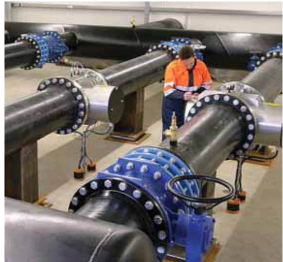
Essen-Horst (Gelsenwasser), Germany 4x DVGW-validated Berson InLine + 15000 4240 m 3 /h
